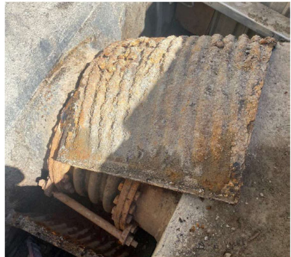
48" Primary Effluent Pipe – Exterior
