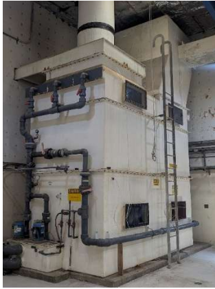
Headworks odor scrubber
