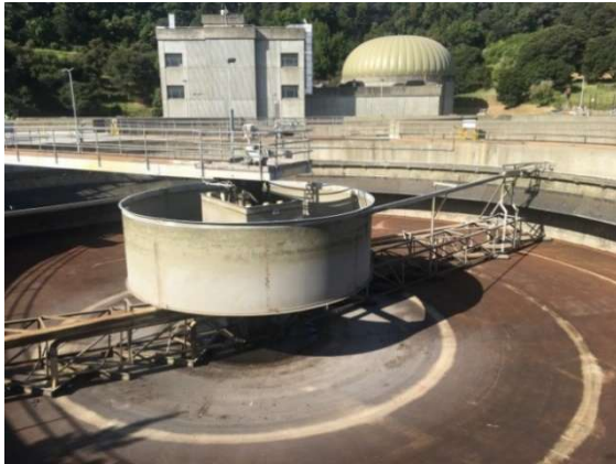
Secondary clarifier internal equipment
