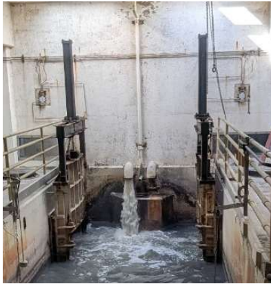
San Rafael and Ross Valley influent gates
