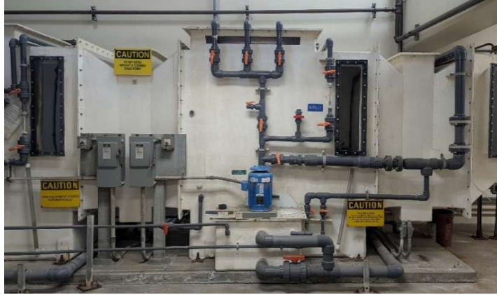
Solids Handling Building odor scrubber
