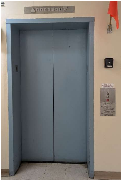
Solids Handling Building Elevator
