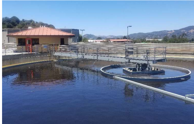
Secondary clarifier in operation
