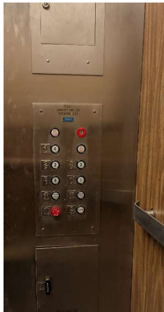
Elevator Control Panel
