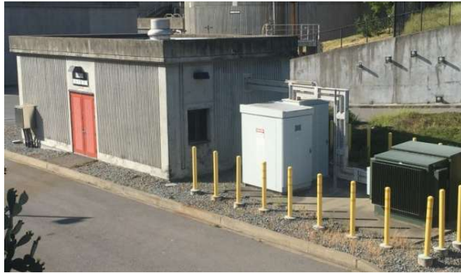
Switchgear building and transformer
